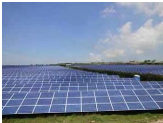
The 5MW Trefullock solar PV farm, Cornwall
