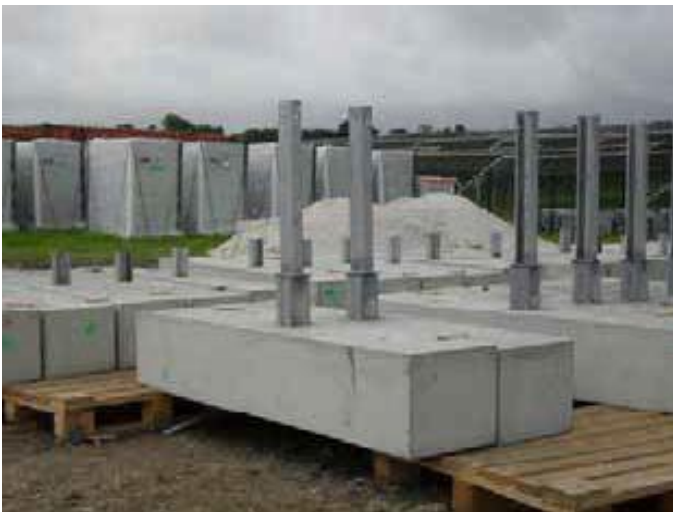
Where there are areas of archaeological interest, and therefore a need to avoid ground disturbance, the use of pre-cast concrete anchors should be considered, as shown here at the 5MW Trefullock solar PV farm in Cornwall
