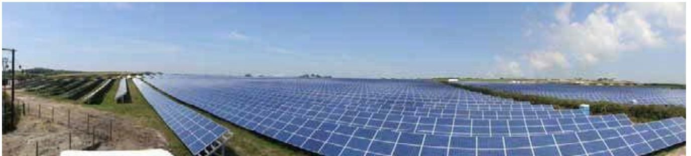
Solar PV facility adjacent to Saarbruecken airport
